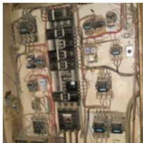
Although this looks dangerous, the actual hazard is low
