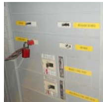
Clean and organized but an extreme hazard is lurking
